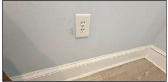
2. Visible growth at wall outlet
