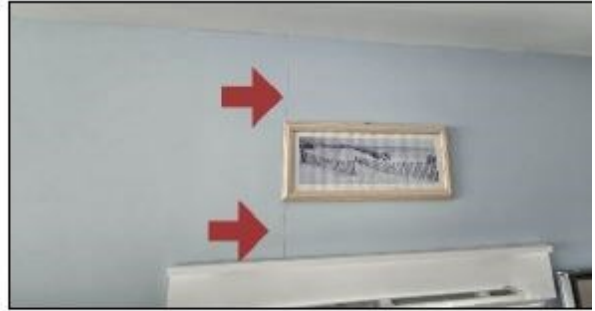
10. Crack in drywall
