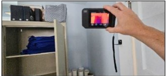
20. Moisture noted at drywall around plenum
