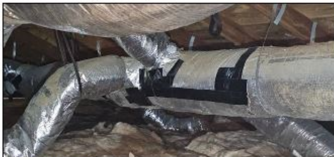
45. Ductwork repaired with improper duct tape
