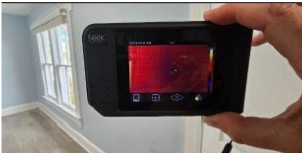
Moistuer in wall beside window
