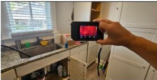
Moistuer behind wall
