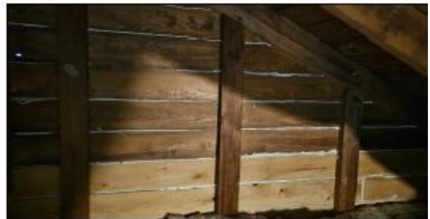
38. Gaps between wood siding
