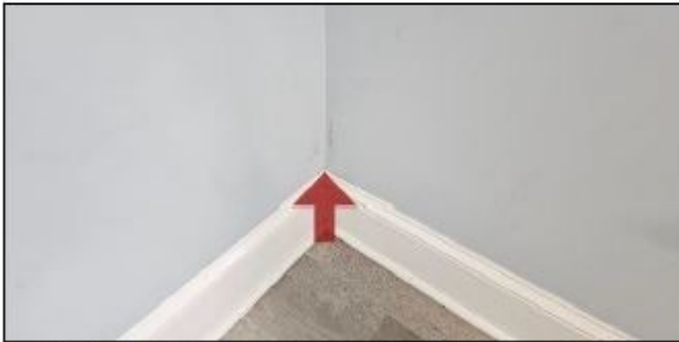
3. Visible growth at corner of wall
