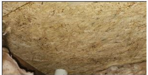
81. Visible growth on subfloor
