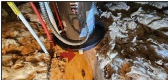
43. Drain line capped - improper
