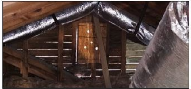
42. Gaps in siding - no wall sheathing installed
