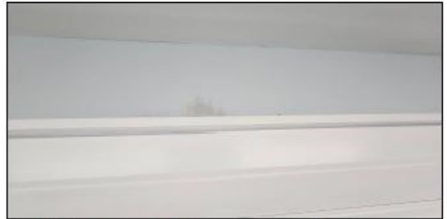
4. Visible growth or infiltration above window
