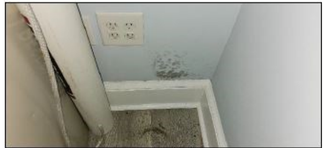
22. Visible growth on drywall near plenum
