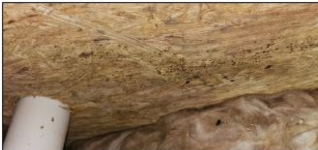
82. Visible growth on subfloor
