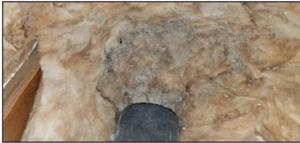
41. Discolored insulation should be removed
