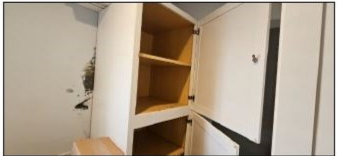
28. Visible growth on cabinets
