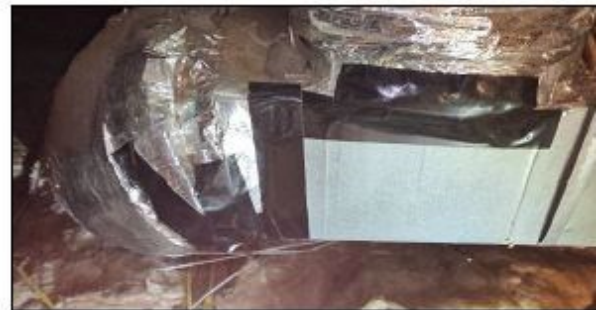
44. Ductwork repaired with improper duct tape
