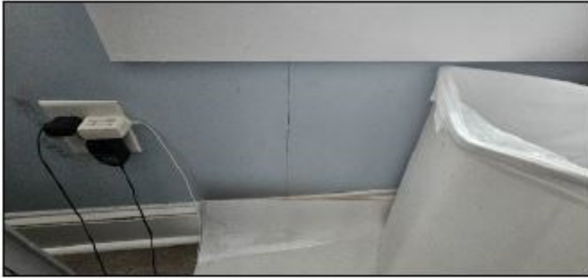
9. Visible growth at baseboard
