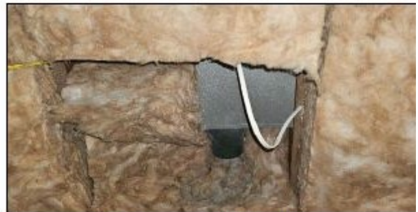
40. Exhaust fan not exhausted to exterior
