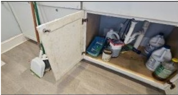
Visible growth on cabinets
