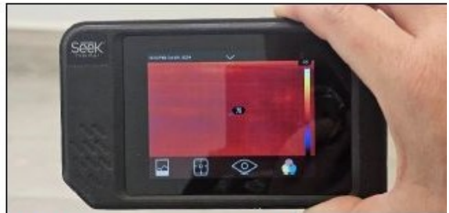
32. Moisture in wall above baseboards
