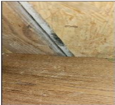
64. Microbial growth on drywall
