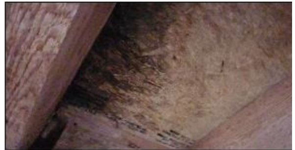
71. Wet subfloor near HVAC plenum
