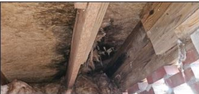
80. Water damaged subfloor
