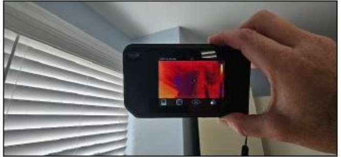
18. Moisture noted at drywall around plenum
