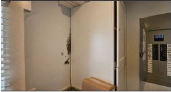
Visible growth on wall behind cabinet
