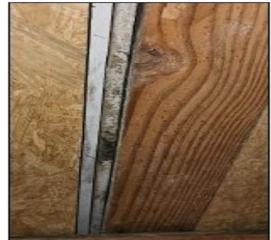
65. Microbial growth on drywall
